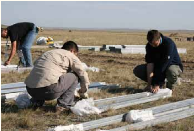
INSPECTORS BUILT THEIR OWN CAMP FACILITIES.
